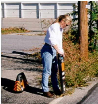
Figure 2.2 - A Pipe Tracing Transmitter/Receiver Being Demonstrated in a Non-environmental Remediation Work Area (Photo courtesy of Enviroscan, Inc.)
